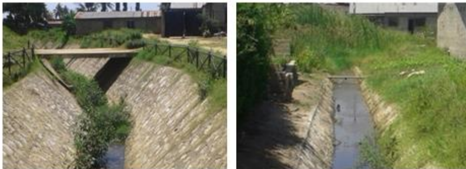
Figure 4.3: The condition of the existing drains where the feeder drains are to be connected
