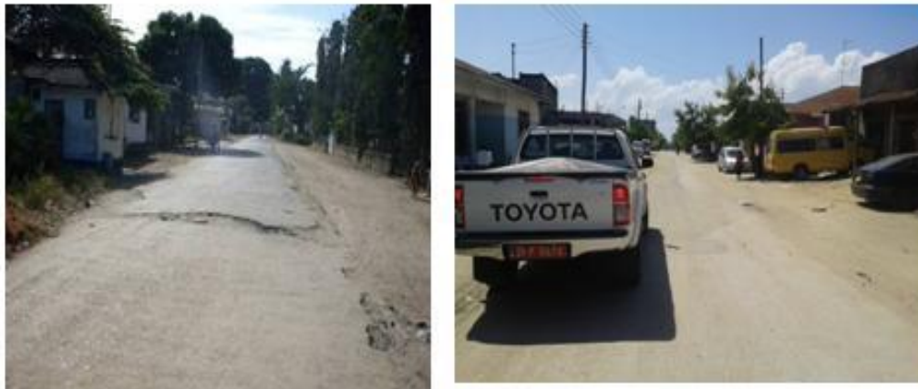
Figure 4.1: Condition of Jamatkhan road
